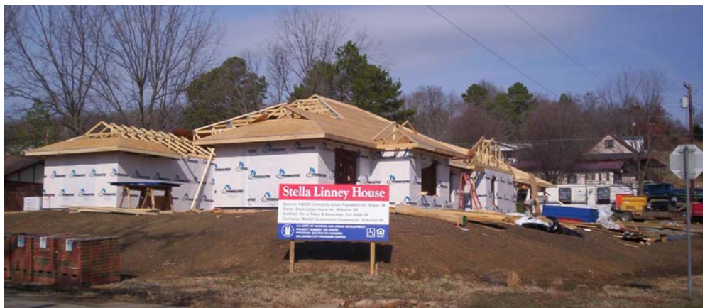
The Stella Linney House, Wilburton, is taking shape as the walls are up and the roof is almost on.. Completion of the house should be by early summer. Photo courtesy of KI BOIS Community Action Latimer County Director Claudia Jeffrey.
